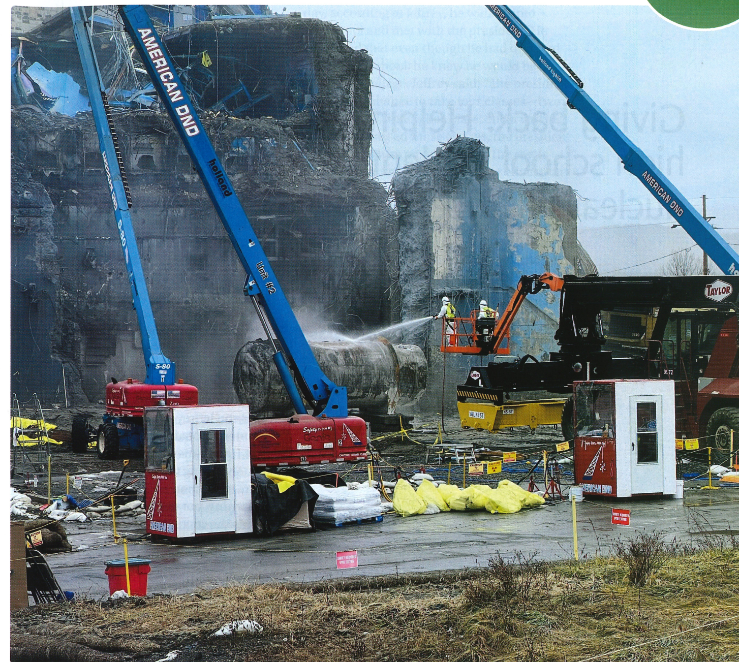
Workers at the West Valley Demonstration Project prepare a large tank for loading after removing it from a liquid waste cell of the Main Plant Process Building. (Photo: DOE)
