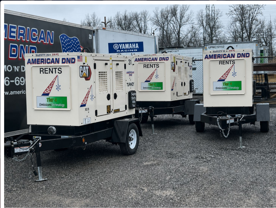
CAT XQ 35 & 60 Generators
